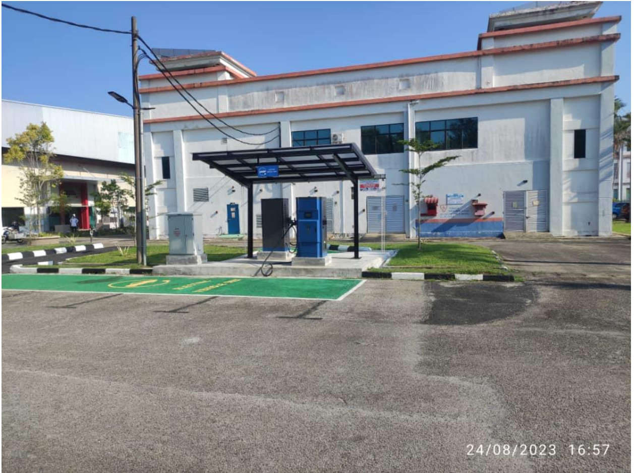
UMPSA Gambang Campus Charging Station
